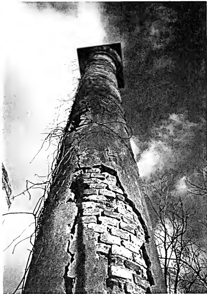
Figure 37: Typical column deterioration
